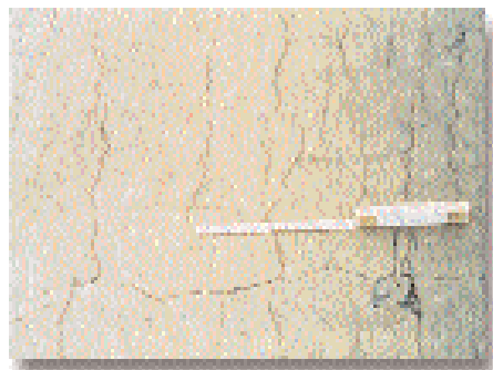
Figure 1: Alkali-Silica reaction causes expansion and cracking of concrete structures and pavements.
