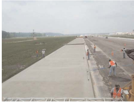
Airport paving at Spirit of St. Louis Airport in Chesterfield, MO, placed with blended cement (Type I (SM)) and Class C Fly Ash added separately.
