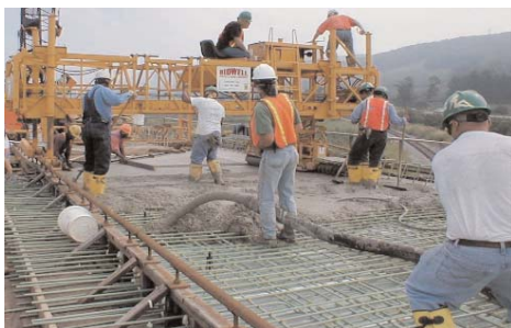
Figure 2: Route 64 bridge deck in Smithburg, MD used high performance concrete with 40 percent slag cement as part of a corrosion-resistant system that extended the predicted life of the structure by 37 years. (Contractor-Joseph Faye Co.; Concrete Supplier-Thomas Bennett Hunter)
