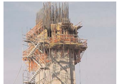
Reliant Stadium (NFL) in Houston, which opened in 2002, used a portland-slag cement-fly ash mixture to achieve both high strength and low heat in its four massive "super columns," supporting the retractable roof.
