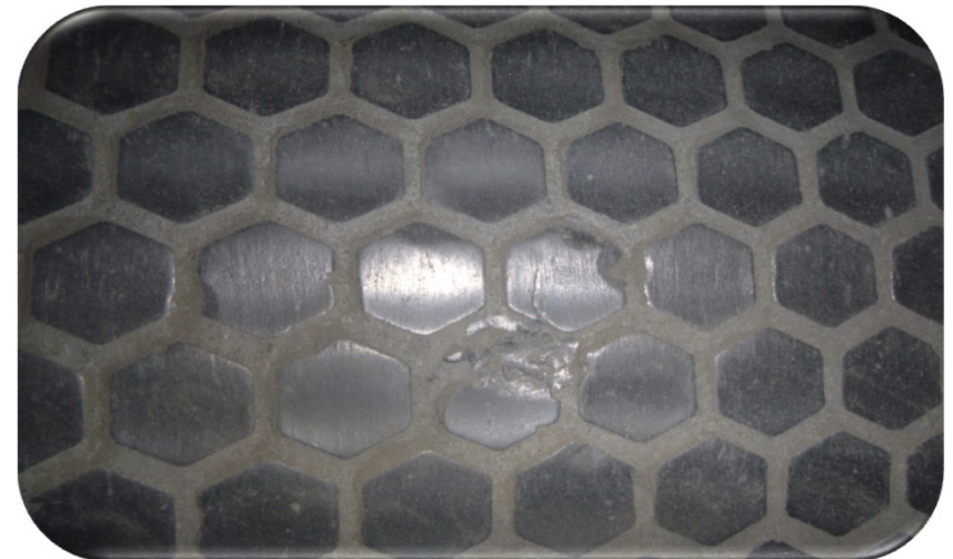
After 12400 hours, wear rate 1,3 to 1,8 mm per 10000 hours of operation
