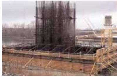
The I-895 Pocahontas Parkway crossing, with massive footings and columns exceeding 16 ft thick, maintained thermal mass concrete specifications and exceeded 5,000 psi 28-day design strengths using a 75 percent slag cement mixture.
