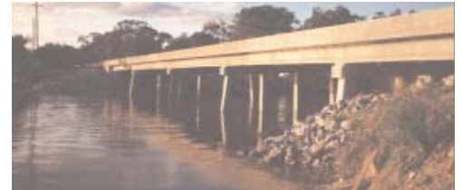
The Charenton Canal Bridge, Louisiana's first HPC bridge deck, achieved a chloride permeability of less than 2,000 coulombs, using a 50/50 percent portland-slag cement mixture.
