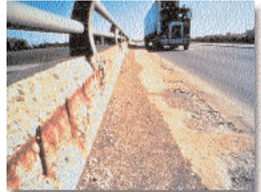
Figure 1: Permeable concrete is a principal reason for concrete deterioration due to reinforcing steel corrosion and other deterioration mechanisms.
