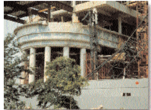
Figure 1: Greening occurred in concrete made with slag cement after forms were removed on the Canadian Chancery in Washington, D.C.
