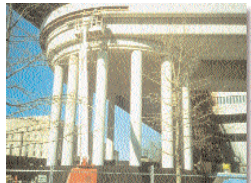
Figure 2: Exposure to sunlight and air allowed the concrete surface at the Canadian Chancery to oxidize and lighten.
