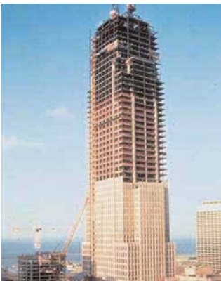
Structural concrete in the Key Tower (formerly Society Tower) in Cleveland achieved over 13,000 psi using a portland-slag cement-silica fume ternary mixture.
