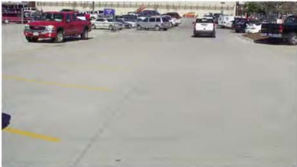
Figure 1: Typical scaling seen on concrete pavement
