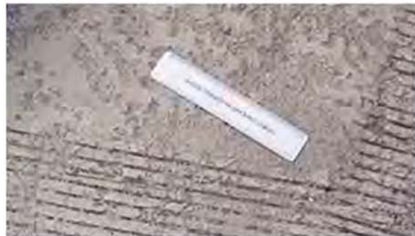
Figure 1: Typical scaling seen on concrete pavement
